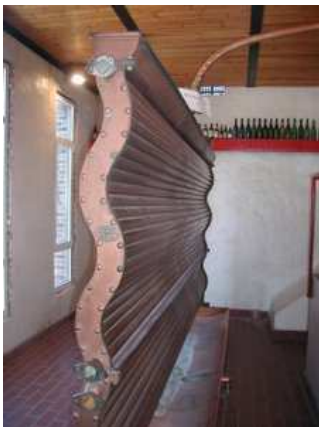
The chiller - after the coolship, the wort was drained down over the OUTSIDE of this contraption, cooling it to fermentation temperature. I asked, but they insisted that no wild yeast cultures were used in this brewery.
